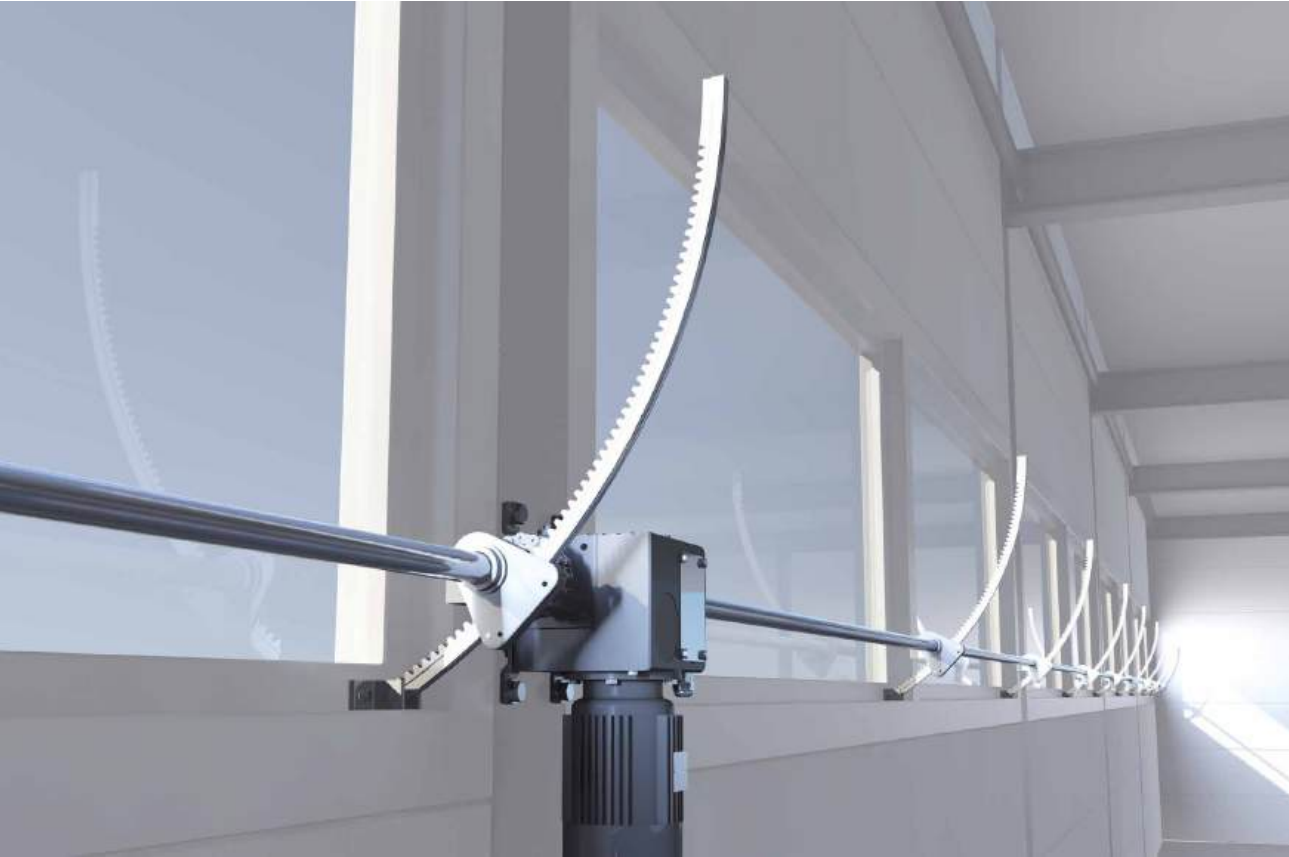
→ Continuous system side ventilation with AZD gear unit, curved rack.
